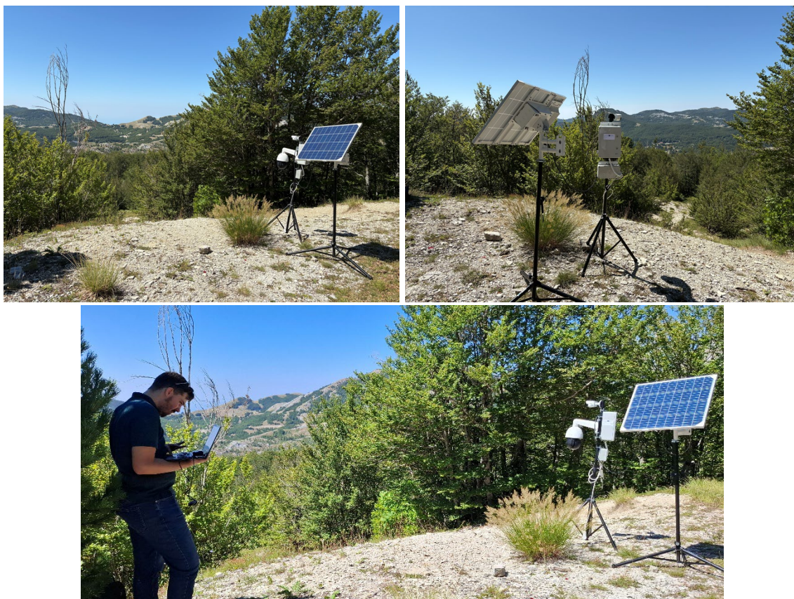
Figure 4. ARCA Mobile WatchStation installed at the Jezerski Vrh monitoring site.
