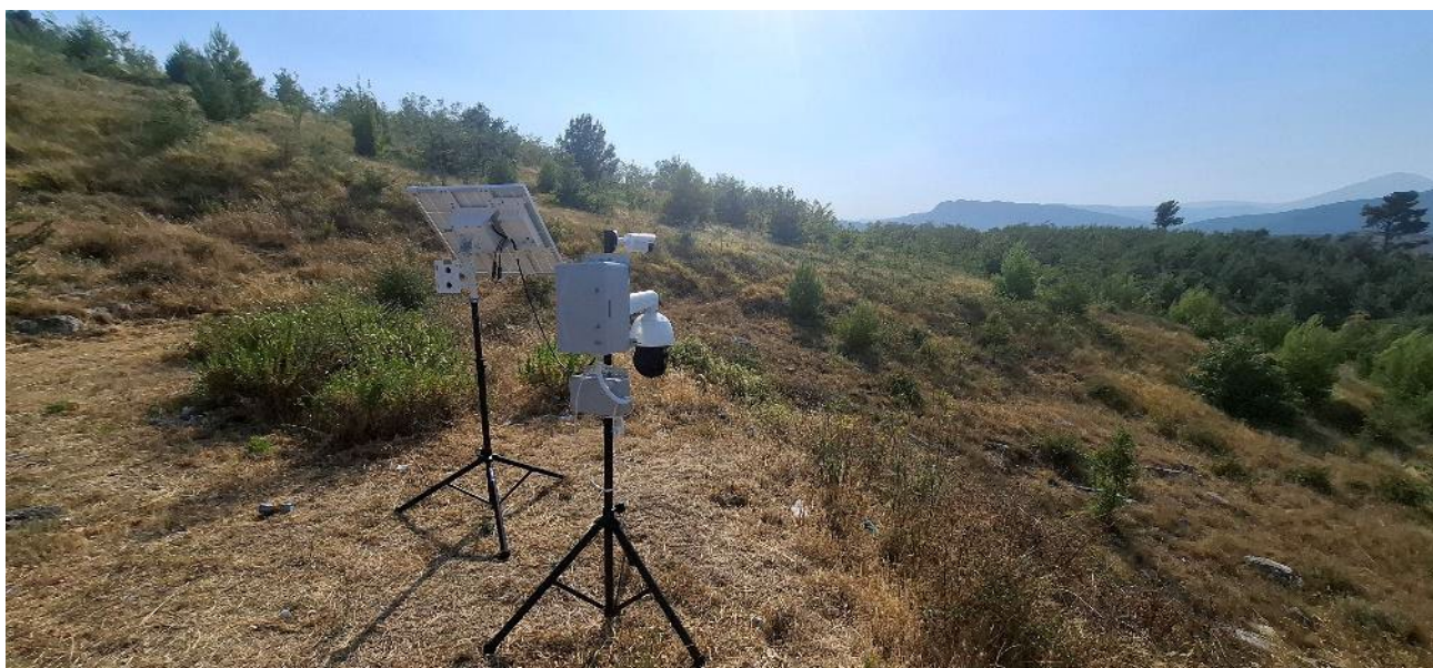
Figure 6. Prototype installation at the Dajbabska Gora test site near Podgorica, Montenegro. The system consists of a photovoltaic power supply, communication equipment, PTZ camera, and thermal camera.
